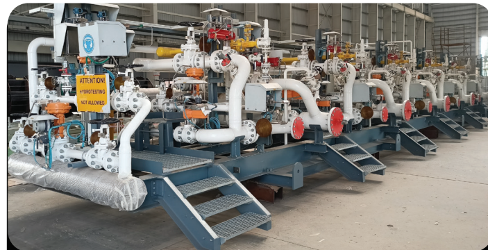
Pressure Swing Adsorber (PSA) Skid for HRRL
