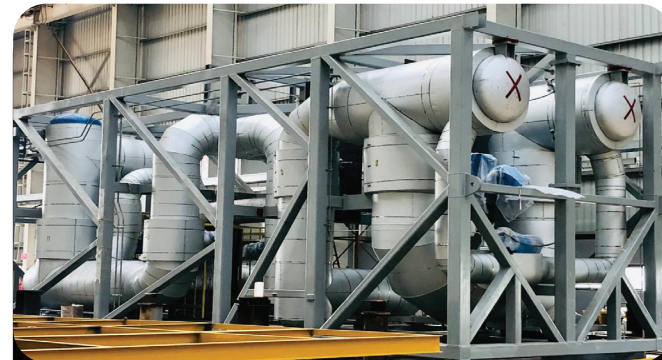
Air Separation Unit-Skid (ASU) for DOMINICAN REPUBLIC-PUEBLO VIEJO
