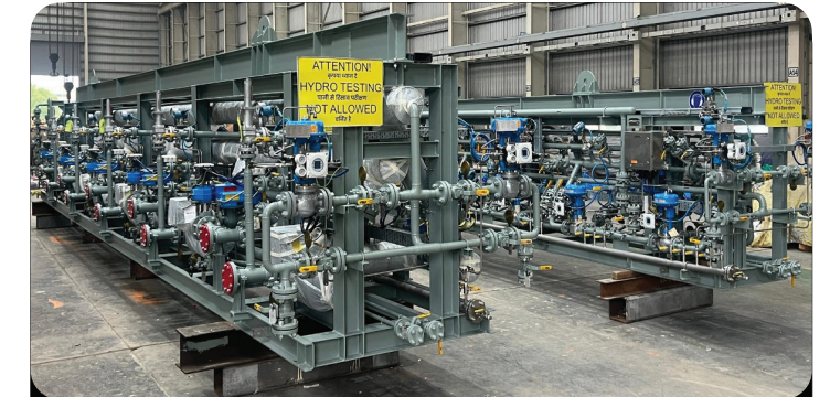
PSA-Skid for Reliance Industries
