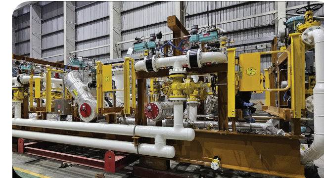
PSA-Skid for Tula Refinery, Mexico
