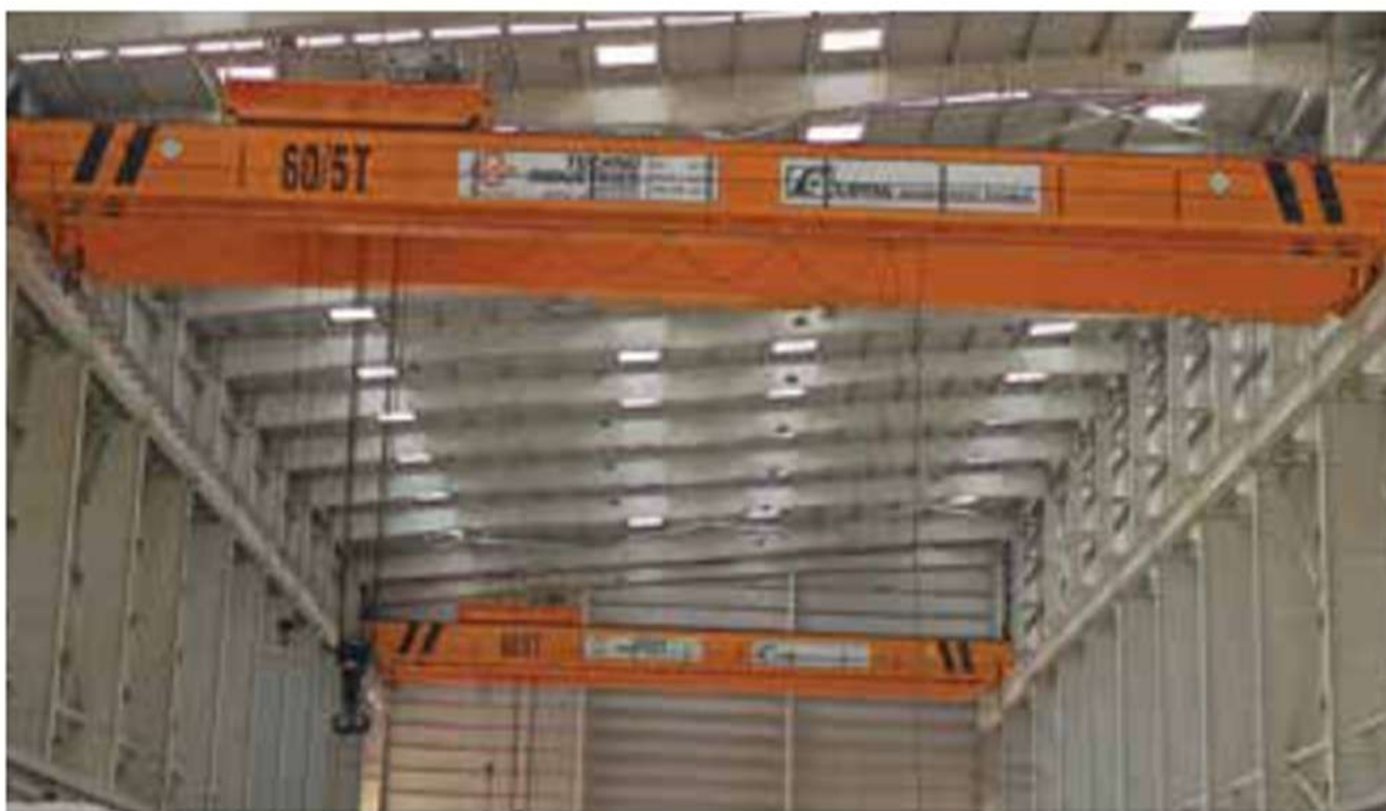
Electric Overhead Travelling Crane (EOT)
